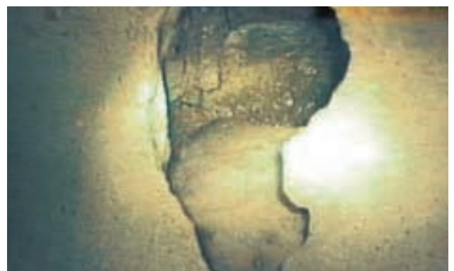
Hole in pipe at joint
