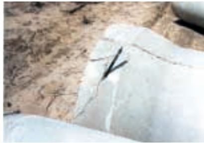
Severe damage and exposed reinforcing steel
