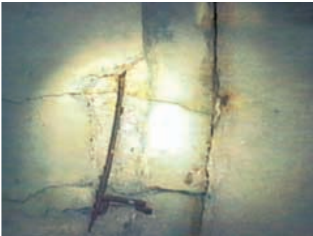
Exposed rebar and cracked bell
