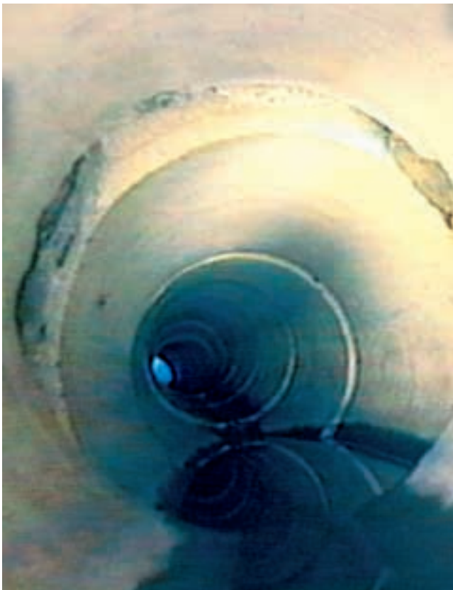
Misaligned pipe - offset joints
