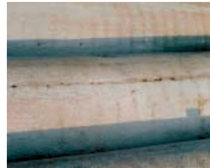
Exposed reinforcing steel
