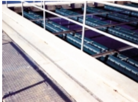
Water treatment plant- corrosion resistance is critical.
